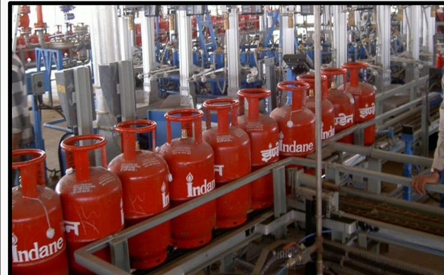
LPG Bottling Plant
