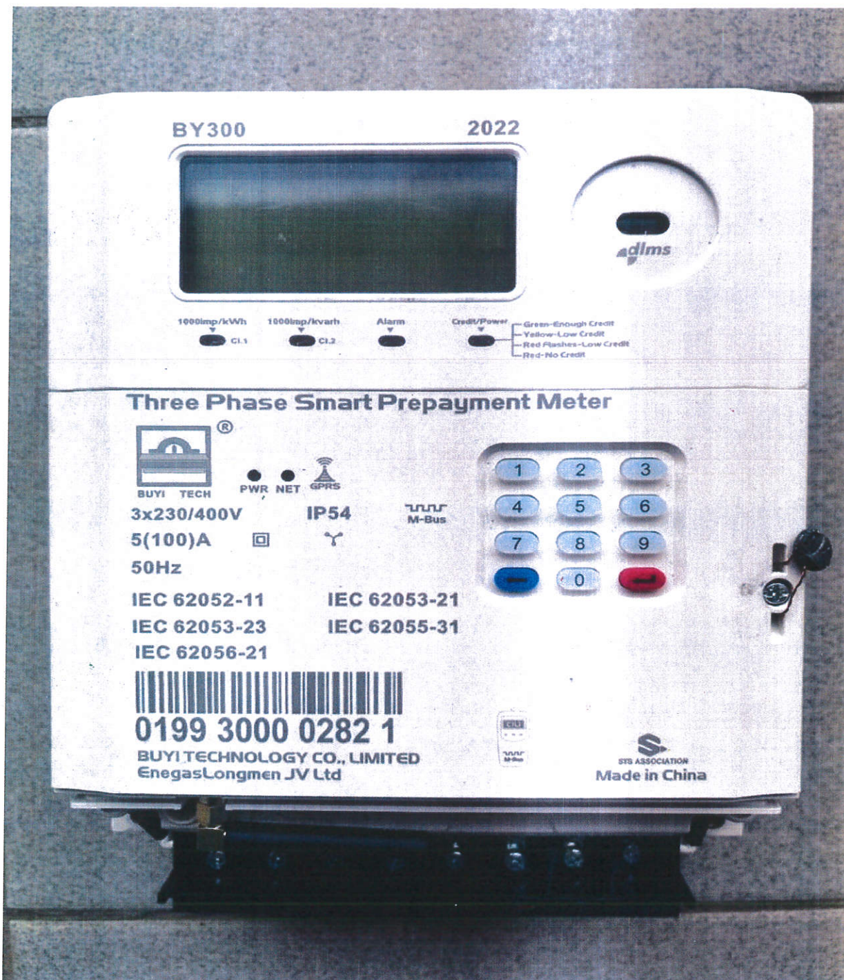
Above is a photograph of BUYI TECHNOLOGY CO. LTD & ENEGASLONGMEN JV LTD Three Phase Four Wire Smart Prepayment Energy Meter with terminal cover open.
